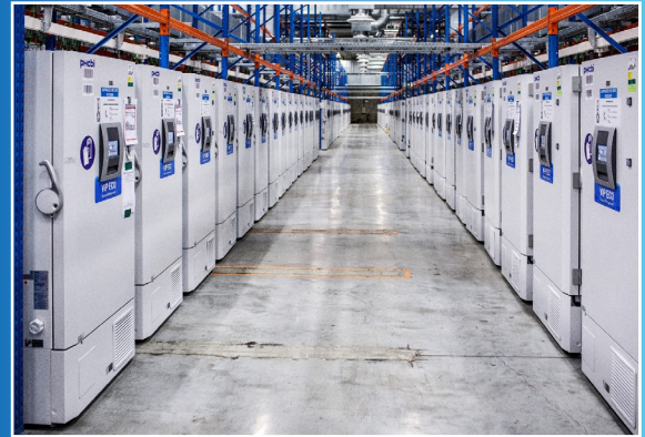
Figure 4. Pfizer “Freezer Farm”
